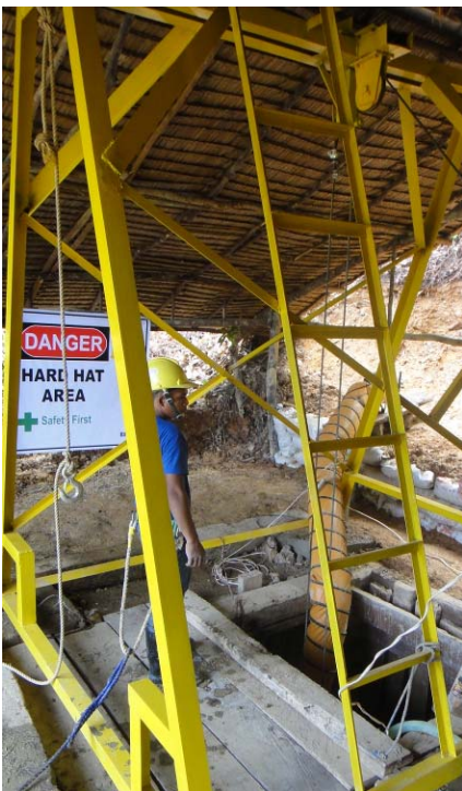
Temporary headframe and hoisting operation to support clean out and refurbishment of No.2 Shaft, Manuel Vein
